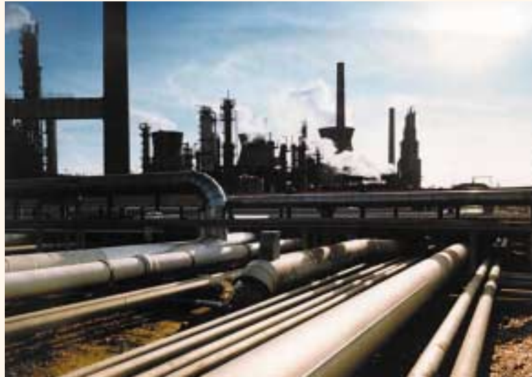
BP's Grangemouth facilities: one of the largest petro-chemical complexes in the UK
